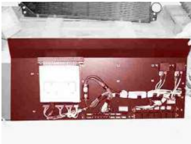
Ceiling switch panel
