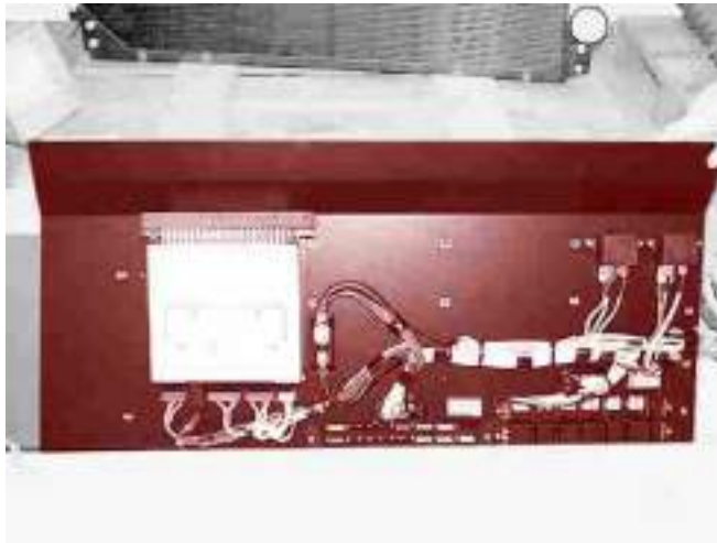
Ceiling switch panel
