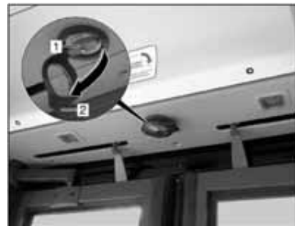
Inside emergency valve – example on city bus
