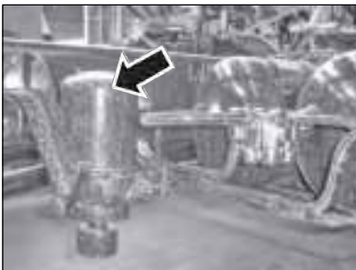
Air dryer heater
