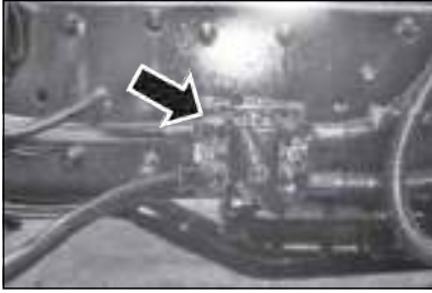
Battery isolator switch
