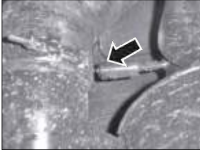
Electric service indicator switch
